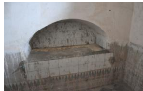
Fig.12 View of the wall niche used to for the hot water supply from the matbah (kitchen) to the hammam
